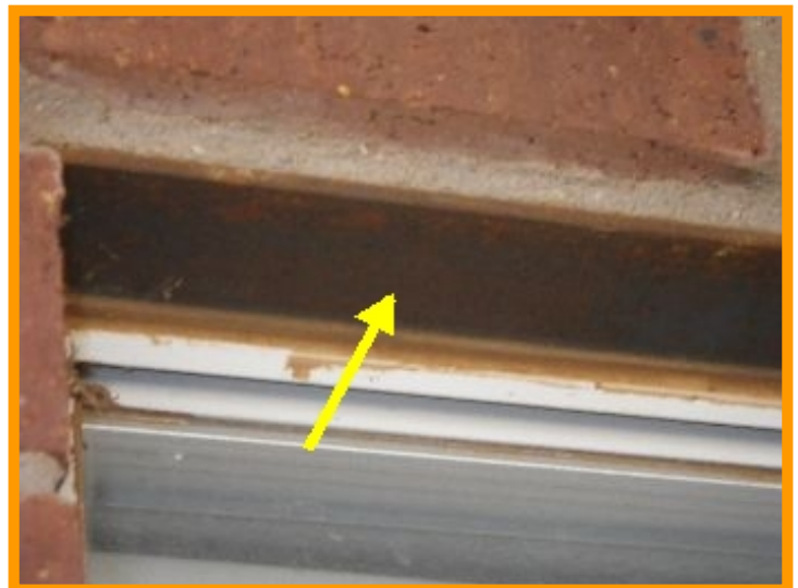
Rust is present at steel lintel support(s) above window, door, or other openings at one or more locations. Repair and painting are recommended to prevent further rusting and possible cracked brick mortar.
