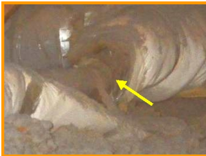
** High Priority Item ** Supply ducts are leaking air at middle part of attic. Repairs are needed.
